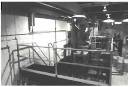
Dust collectors mounted above the test center floor leave room for material and test equipment below.
